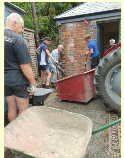
Meanwhile work continued on the french drain around the building. Member Dick Smith's grandsons joined in to help Mike and David.
