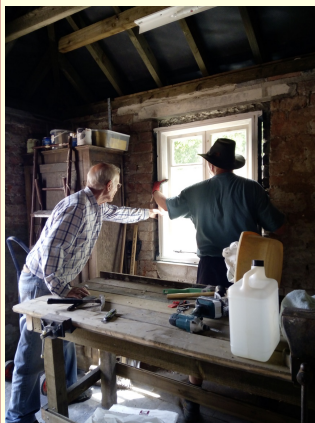
David and Mike securing the window in the left hand side of the building
