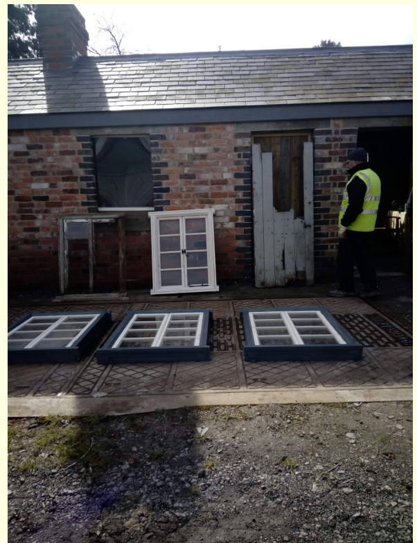
Photo above: Four of the new windows displayed with the original rescued window
